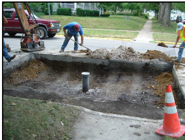
Figure 66 -- Geogrid being placed after the fourth lift and T-section were excavated with backhoe on east side of the trench
