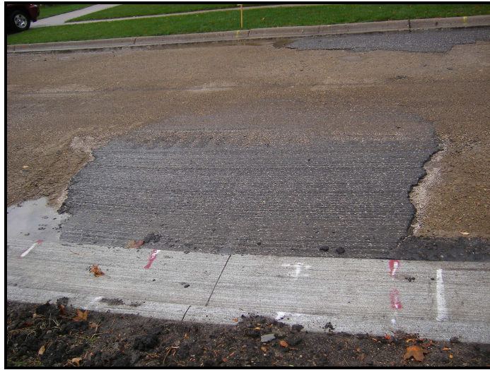
Figure 179 -- Runoff flowing into the trench around the temporary patch
