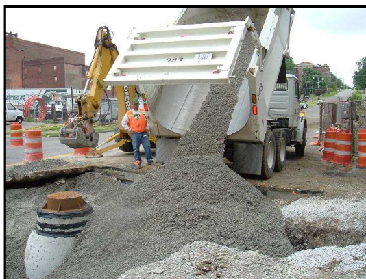
Figure 2 -- Large lift thickness used in utility cut trench backfilling (Schaefer et al.. 2005)
