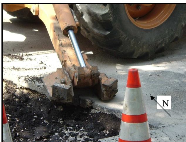
Figure 60 -- Support of the backhoe at the edge of the pavement on the east side of Trench E
