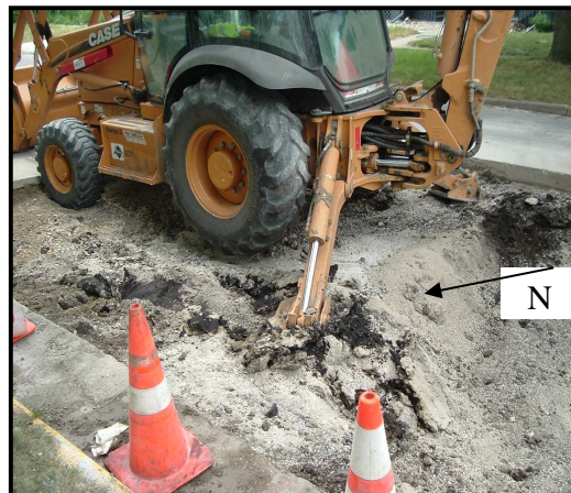
Figure 47 -- Backhoe operating where pavement was removed on the northeast side of the trench
