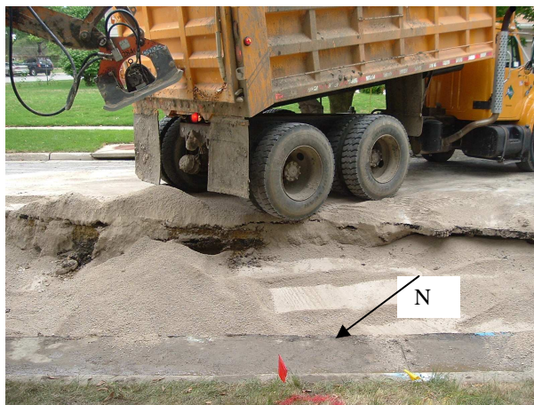
Figure 45 -- Truck backing into Trench A from east side of Trench A with backhoe with attached vibratory plate compactor operating on northwest side of Trench A
