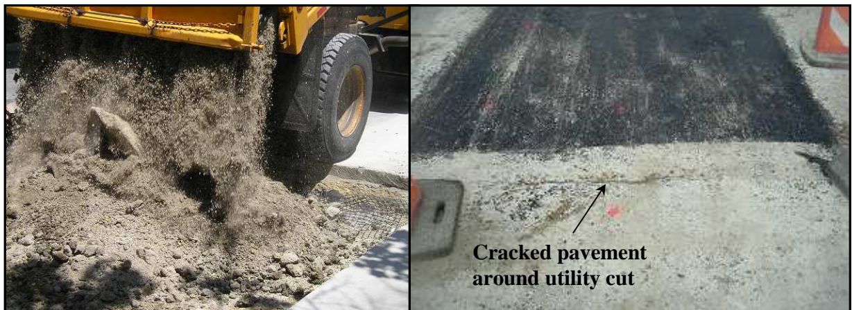
Figure 1 -- Cracking pavement surrounding the utility cut area, because of construction equipment getting too close to the edge of open cut (Schaefer et al.. 2005)
